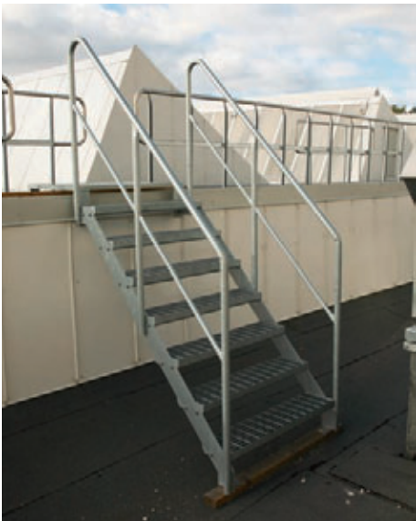
Staircase with stringer of Flat Bar.
